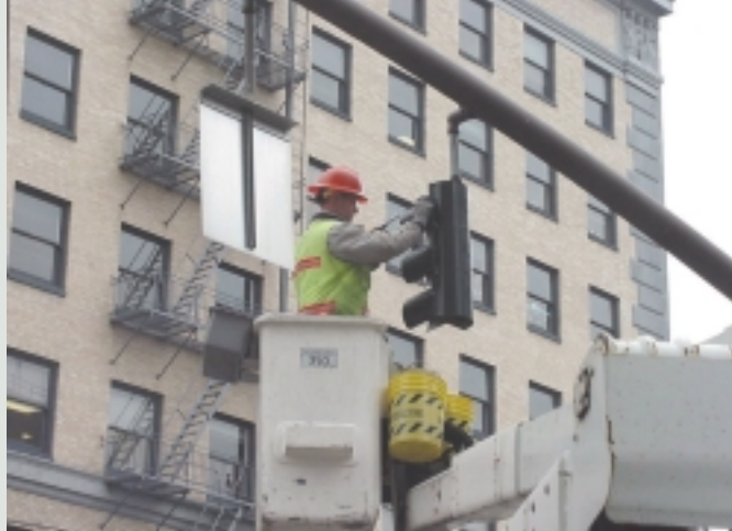
A City-hired contractor installs one of more than 13,000 LED lamps during the fall of 2001.
