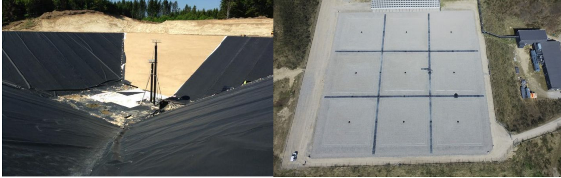
Figure 2-5. 60,000 m 3 (2,118,880 cu ft) “SUNSTORE 3” pit storage in Dronninglund, Denmark, 2013. (SHC Task 45).
