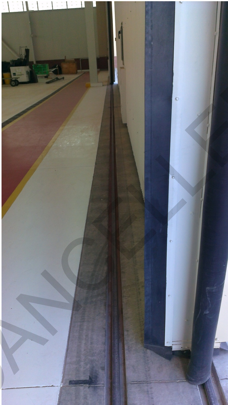
Figure E-12: Sliding Hangar Door Tracks
