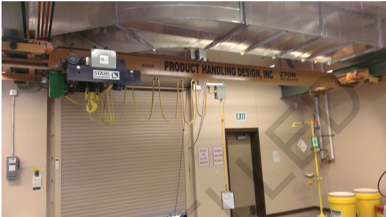
Figure E-11: Overhead Bridge Crane within a Shop
