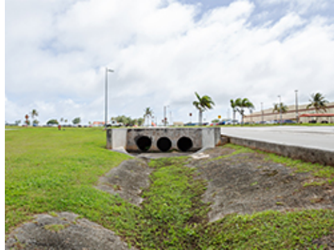
Stormwater Pipe at Street
