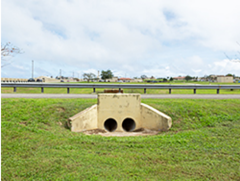
Stormwater Pipe at Street
