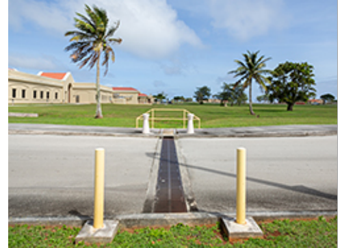
Inlet and Grate
