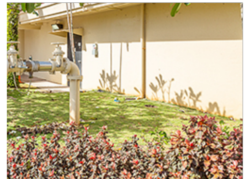
Roof Drainage Directed through Planting Bed
